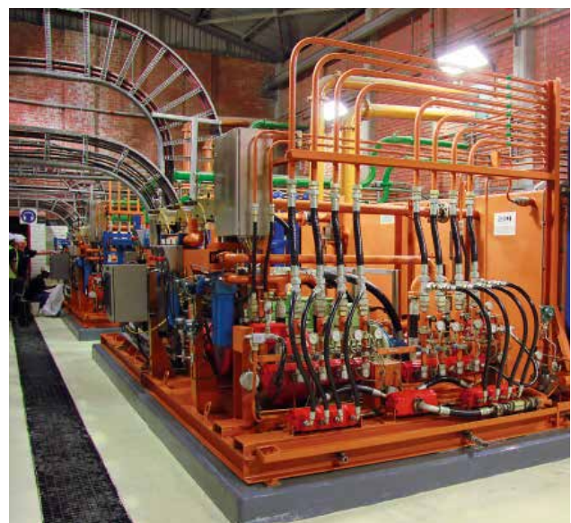
Central lubrication system with GHM Honsberg flow meter, Pressure sensors and temperature sensors.
