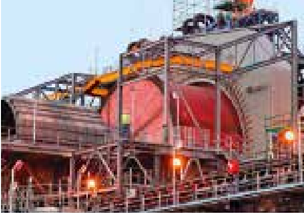
Stone mill in South Africa with large bearing operated via a central lubrication system. The oil volume is measured with VHS equipment of GHM.
