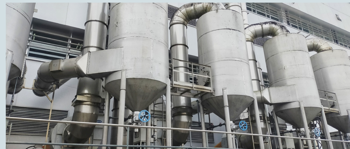
Chemical gas scrubber
