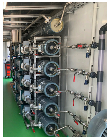
A view into the container, showing the semi-permeable membranes of the reverse osmosis system.
